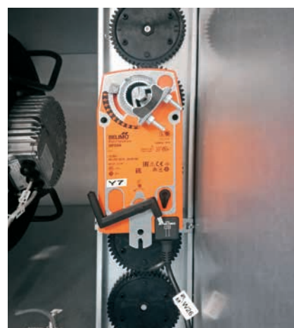
Figure 54: Actuator for the fresh air and exhaust dampers.
