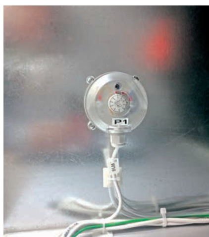
Figure 49: Differential pressure switch for fresh air or extract air filters.
